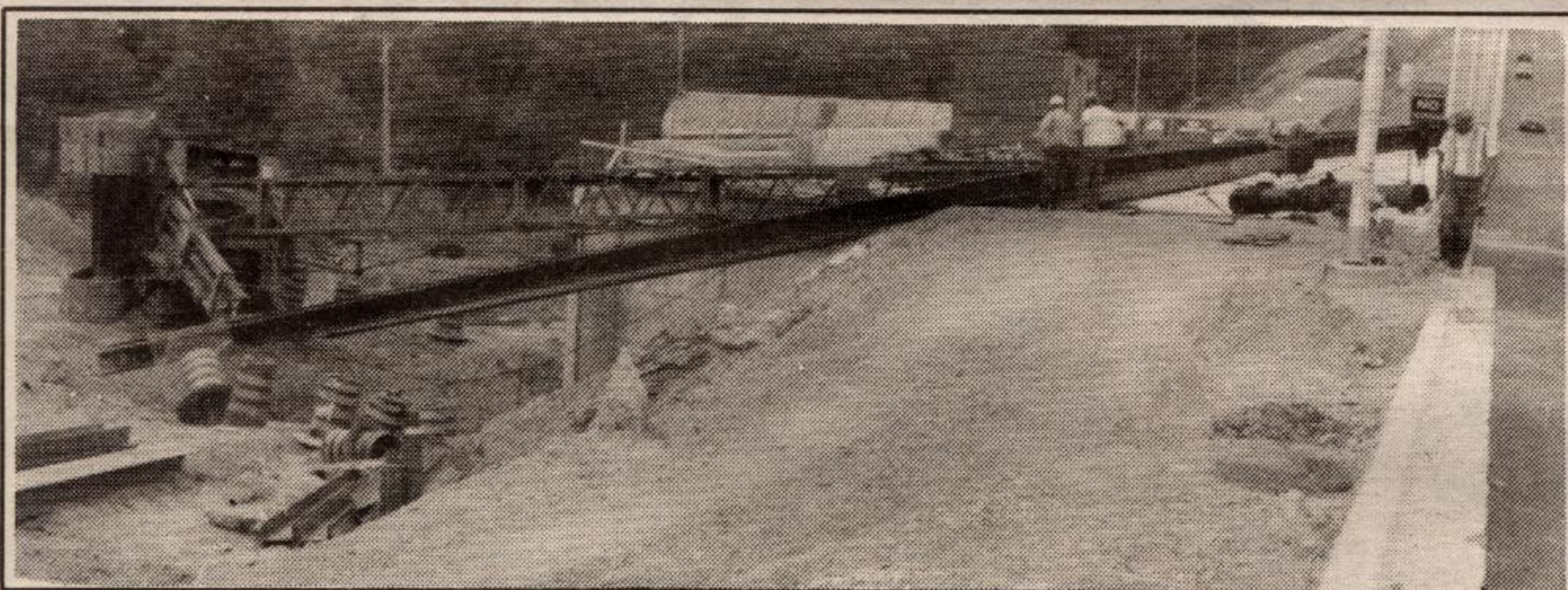
CRANING FOR A VIEW! Nobody was injured last Monday when a pile driving crane toppled over on the Hungry Hollow Bridge. The Ministry of Labour has issued a stop work order while it investigates the accident. (Jamie Harrison photo)
