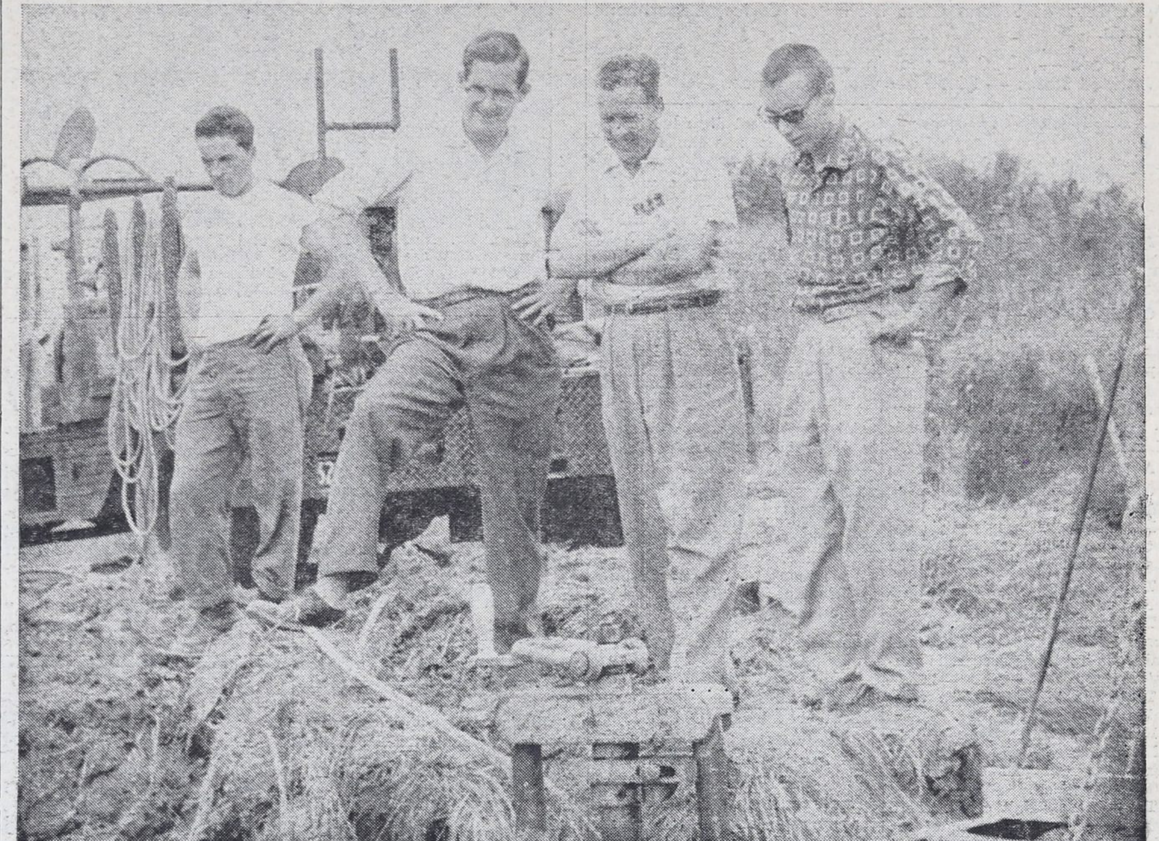
Northern Ontario Natural Gas company performed a major operation on feed lines into Haileybury, rerouting the line and placing a protective casing around the main where it will pass under the Tri-town bypass. Division engineer Bob Snyder, in charge of the project, District Sales manager Bud Wynn and salesman Bob Hinds look over the giant stopper valve used in the operation.
