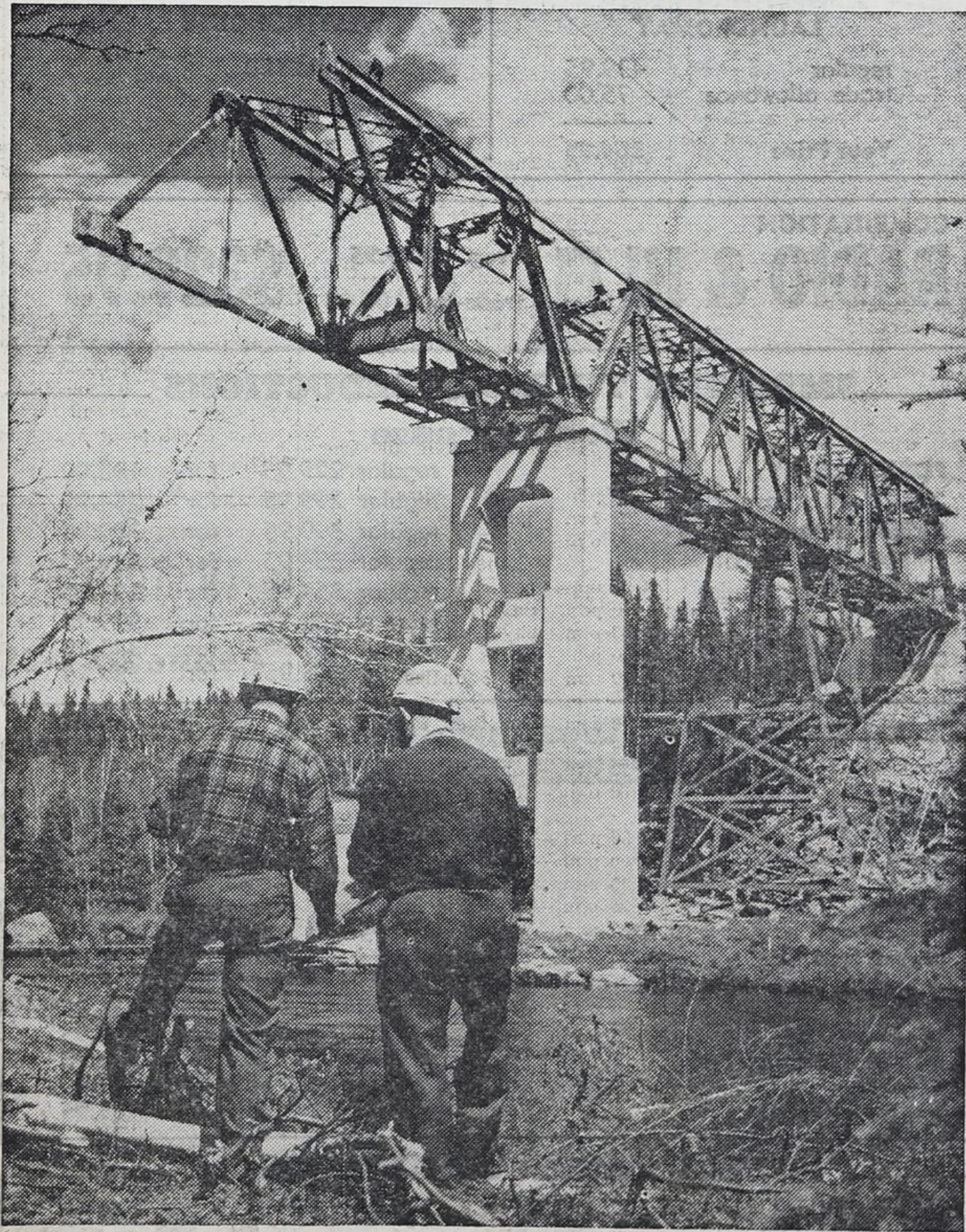
BRANCH LINE NEARS COMPLETION — One of the most difficult construction problems faced by Canadian National Railways' engineers in the building of a new 294-mile C.N.R. branch line to link mineral-rich Northern Quebec with the industrial areas of the
