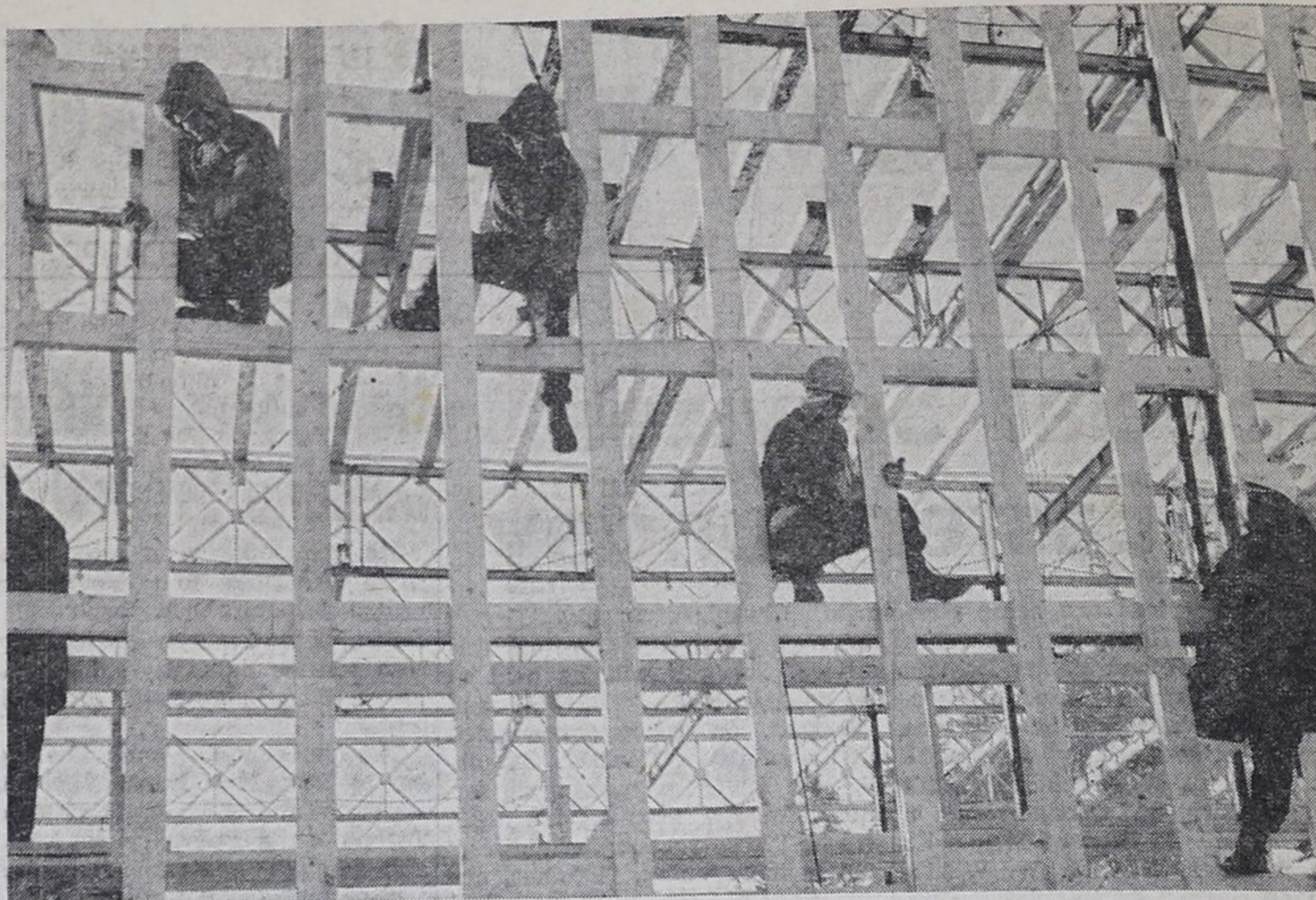
These agile, sure-footed gentlemen find themselves going up in the world as they build the framework of a structure over one of the diversion sluices at Ontario Hydro's Red Rock Falls Generating Station. Located on the Mississagi River, some 12 miles northeast of Thessalon, this new, two-unit plant is expected to have a capacity of 38,000 kilowatts and to be in service by late 1960. It is one of four important developments now being built by the Commission in northern Ontario to safeguard and improve the power supply in that part of the province. The estimated cost is approximately $19 million. — Ontario Hydro Photo No. RR-257
