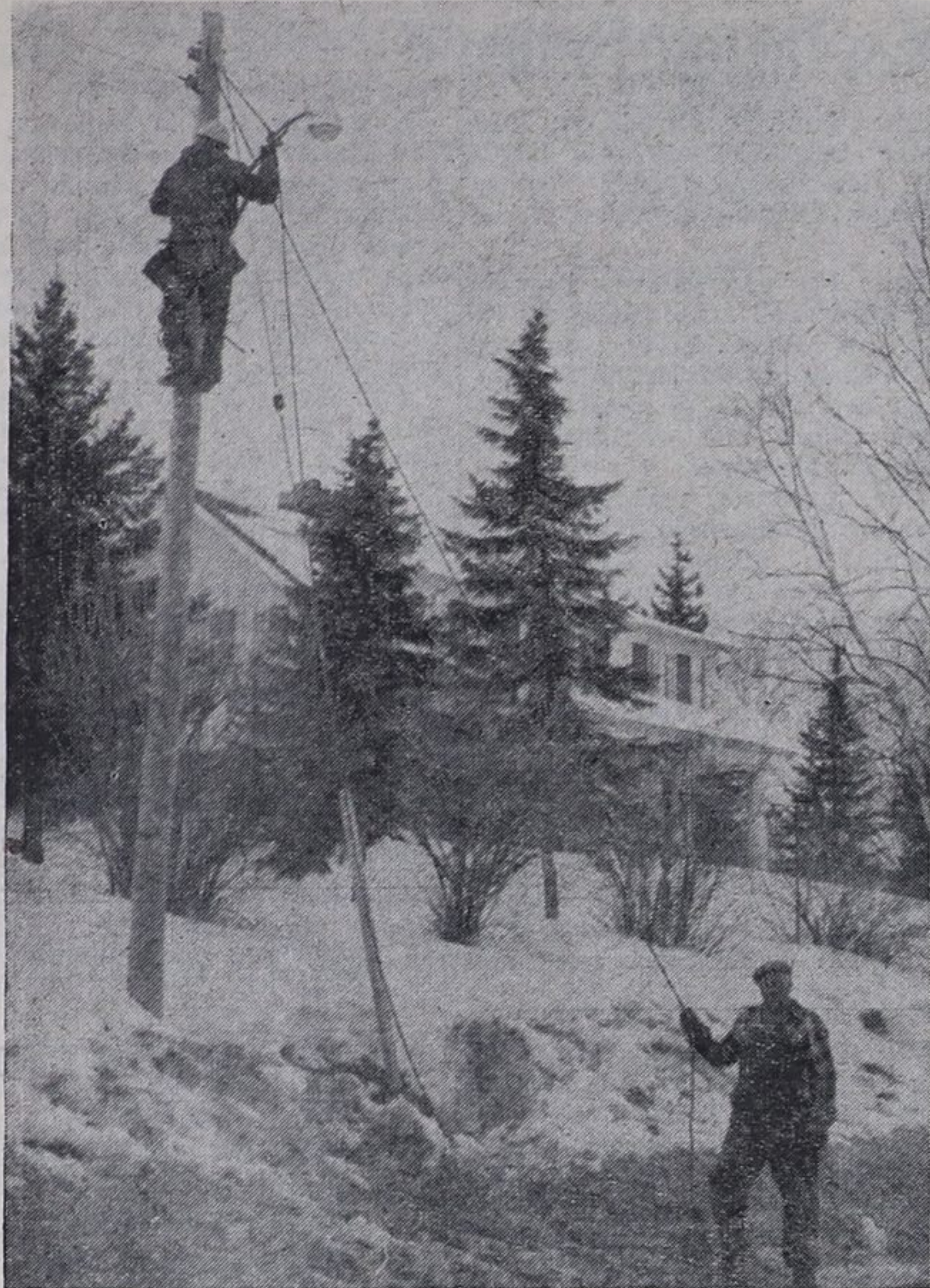
Hydro officials have announced that a general rehabilitation of street lighting facilities is taking place in the Tri-town area. The improvement of street lights is to take place over a period of months, the main change being the transformation from the old series circuit wiring to the more modern multi-circuit wiring. The lighting source is being changed to the global type. Above members of a hydro crew are completing the exchange along the Lake Shore Road in Haileybury.
