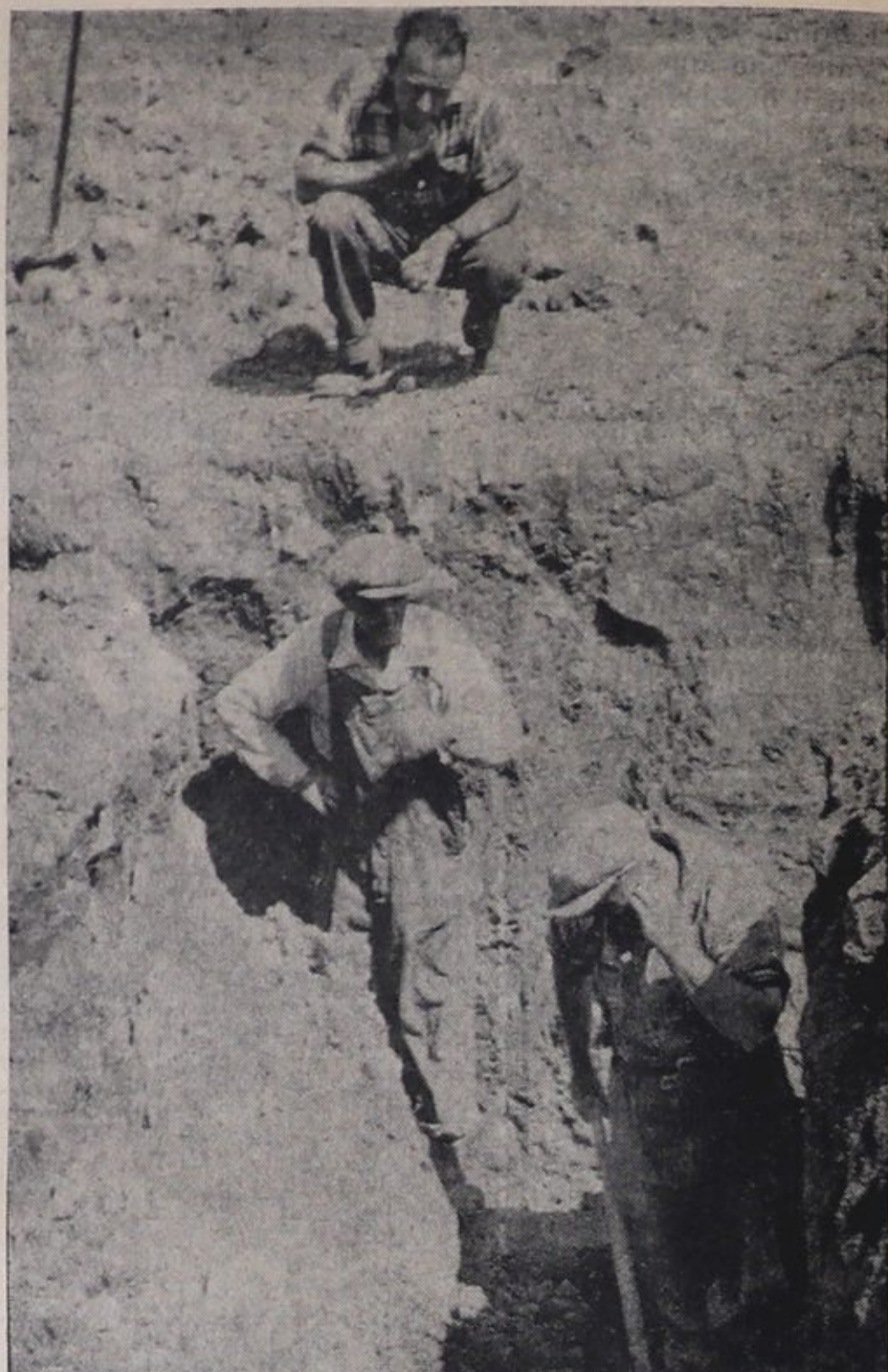
The town gang can claim to be the muddiest men in Haileybury these days. Installation of the new water lines at the south end of Haileybury are nearing completion. Above, Verdon Cooke takes time out to swat a pesky fly. Albert Palmer looks on, while sidewalk superintendent Hilliard Cooke heckles from the sidelines.
