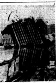
The above photo shows the Ogville elevator after the foundation gave way and the structure slid into the Kaministiquia river on May 28, 1906. The machinery of the big Ogville mill was turned over yesterday for the first time and within a week will turn out 3,000 bags of flour per day," stated the story describing the event.
