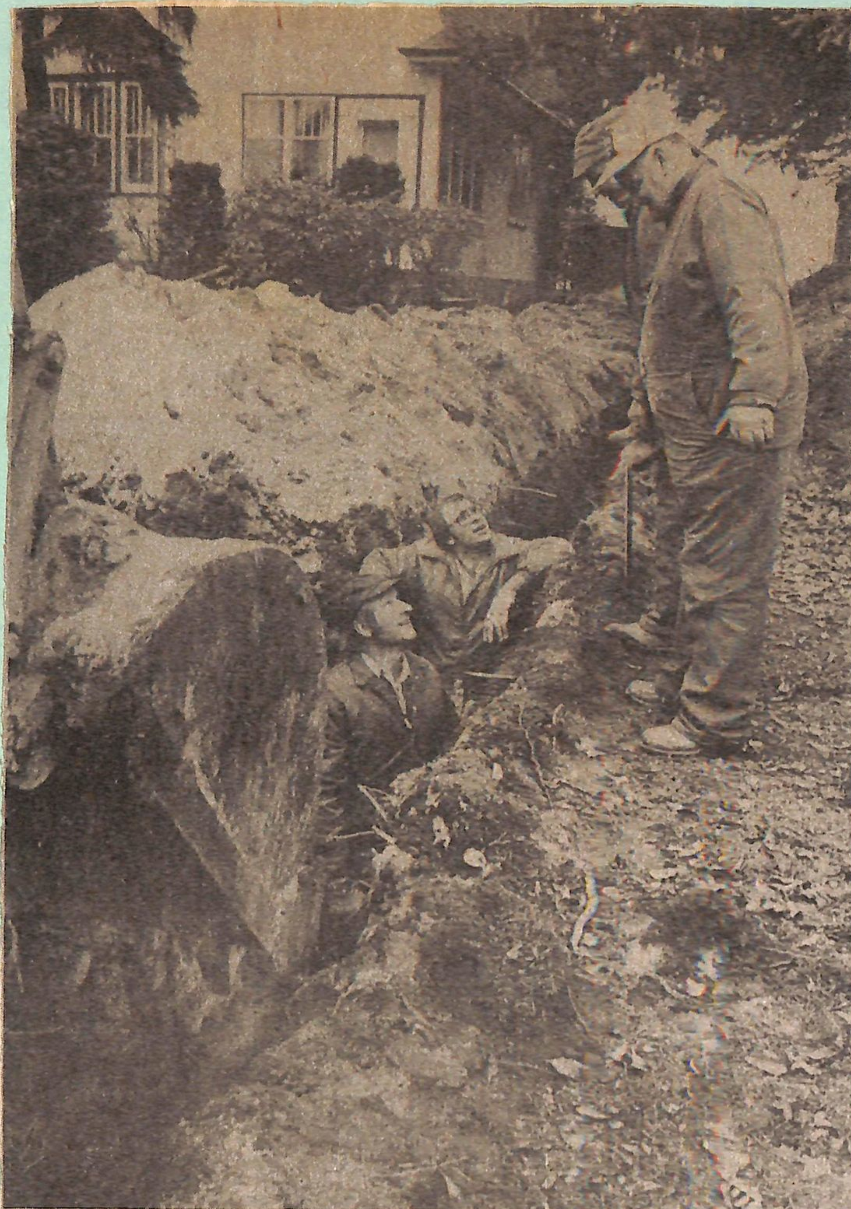
WORK ON THE RECENTLY purchased Lakeside water system began last week. Replacing 2-inch water lines with 4 ft. 2-inch mains are from left: Ward 4 councillor Wayne Smith, member of Lakeside's water committee Gerald Lichty, contractor George Heron and Zorra Tsp. employee Bud Haslen. (Staff Photo)
