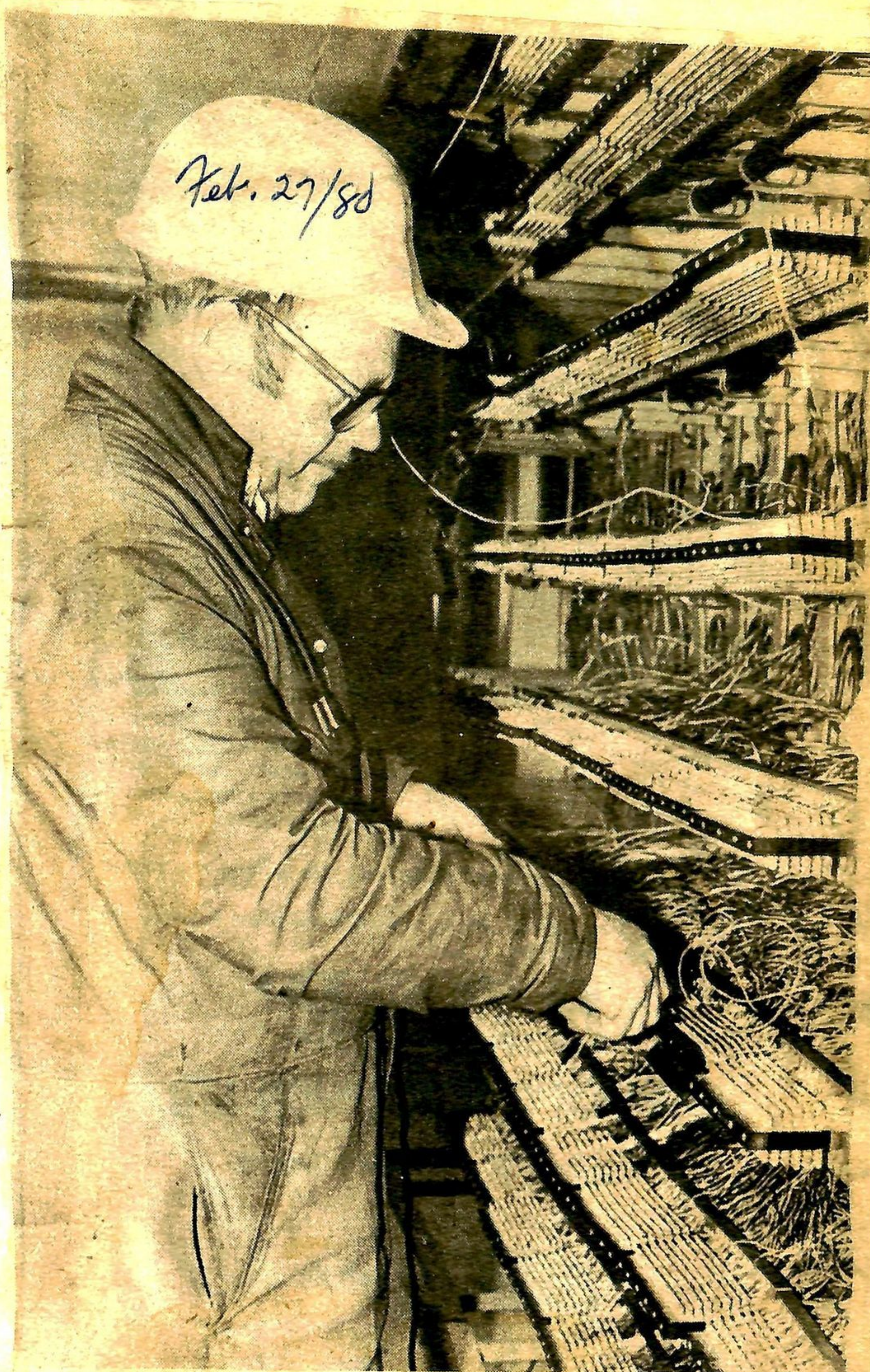
Vic Moore, an employee with the North Norwich Municipal Telephone System in Burgessville, hooks up a new telephone connection at the main frame. He has been with the company for about 30 years.
