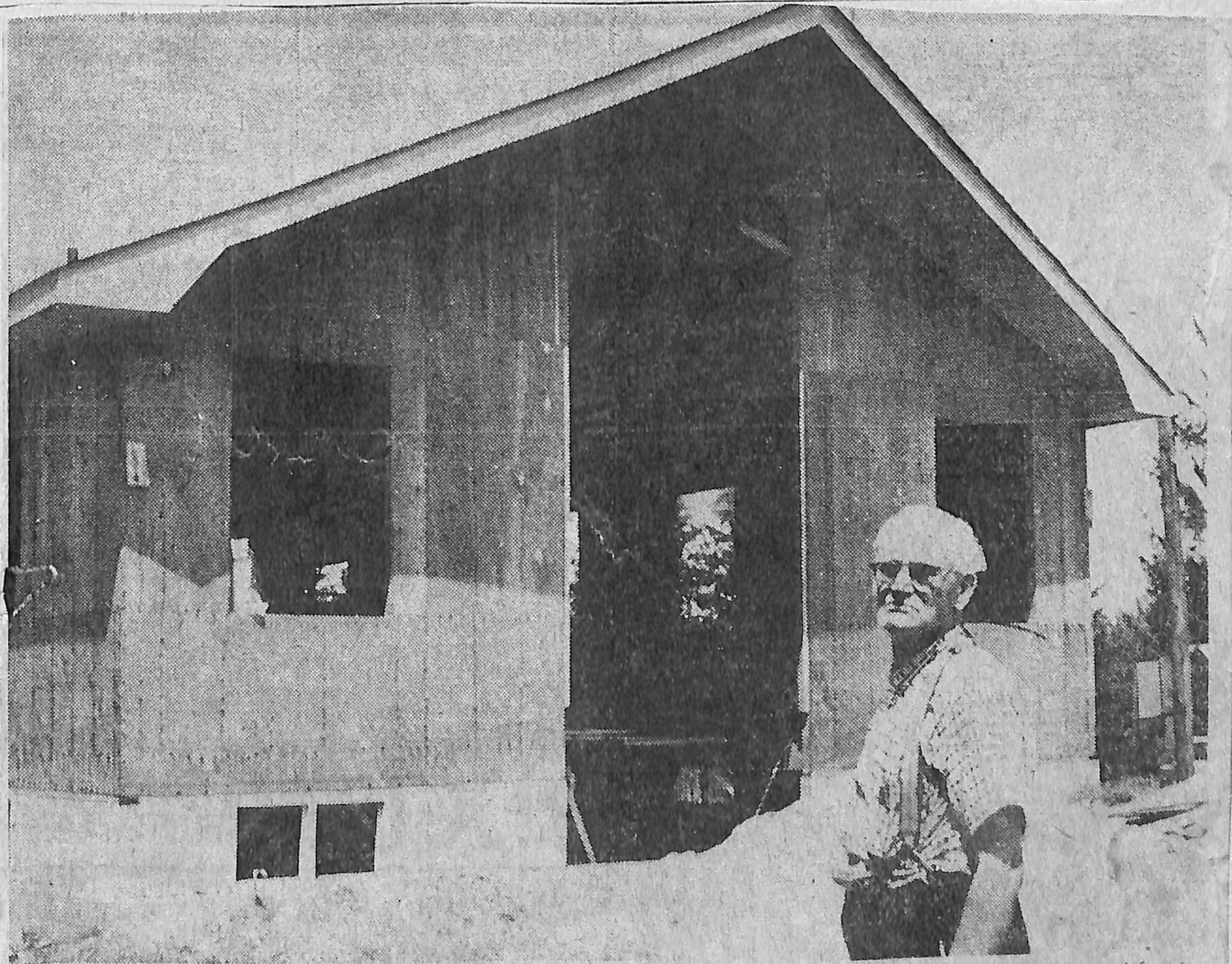
NEW CHURCH RISES —A church to replace the Harrington Presbyterian Church, destroyed by fire, is rising on the site of the old one. Shown in front of the church is John Morrison, who was "too young to help when the old church was moved, and too old now to help with the new building."
