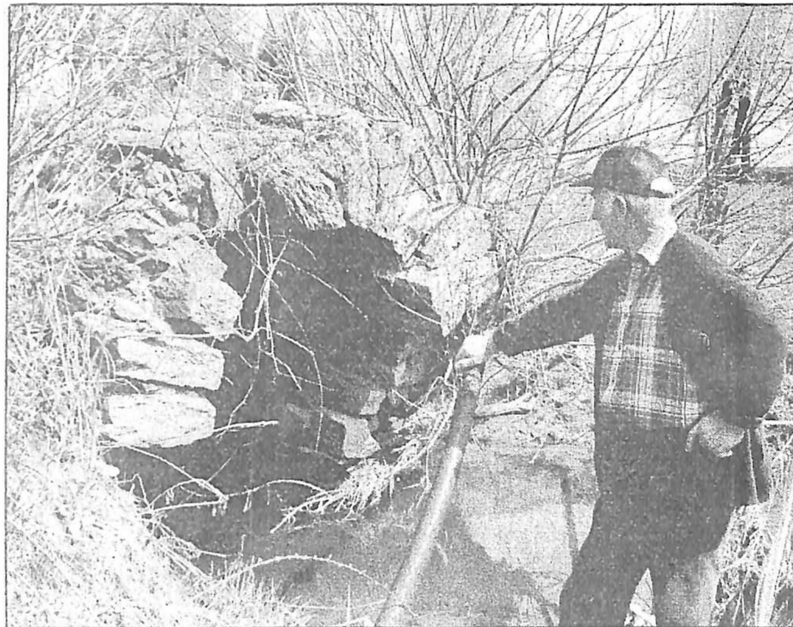
Long-time resident Scotty Robb fears time is running out for the hamlet's stone-arched bridge. Time has taken a heavy toll on the rare structure which dates back to the 1850s.
