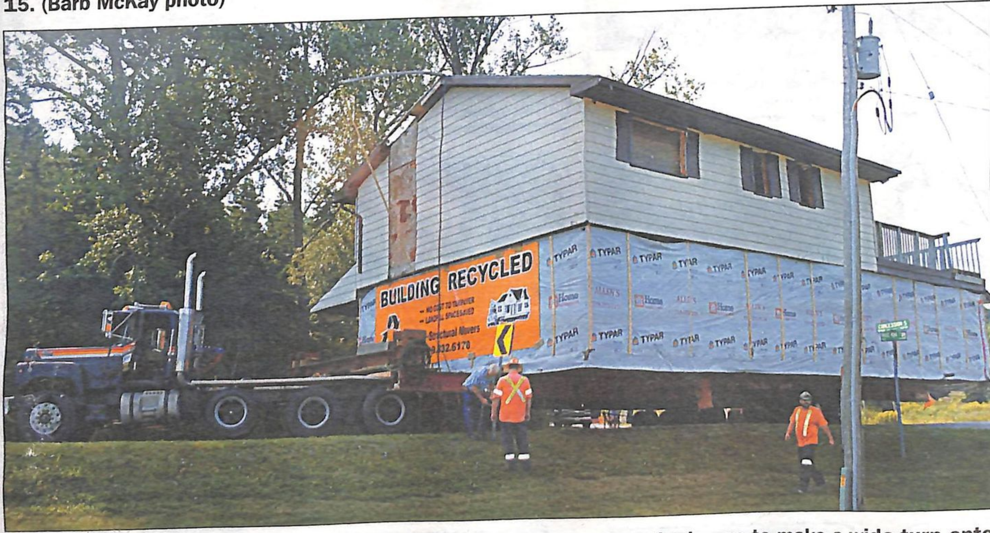
Ken Jackson helps remove a road sign in order for the truck carrying the house to make a wide turn onto Bruce Road 23. (Barb McKay photo)
