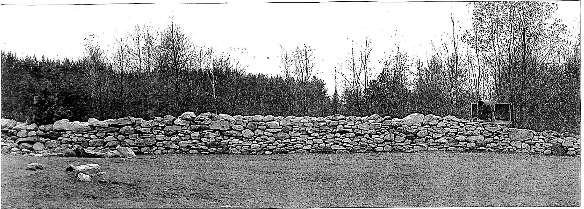
It's not exciting work and it's not fast work. It's boring, dull and deadly. And I rather enjoy it," says the stone fence builder. Wendell Sedgwick is barely visible as he lays stones at the far right end of the fence.
