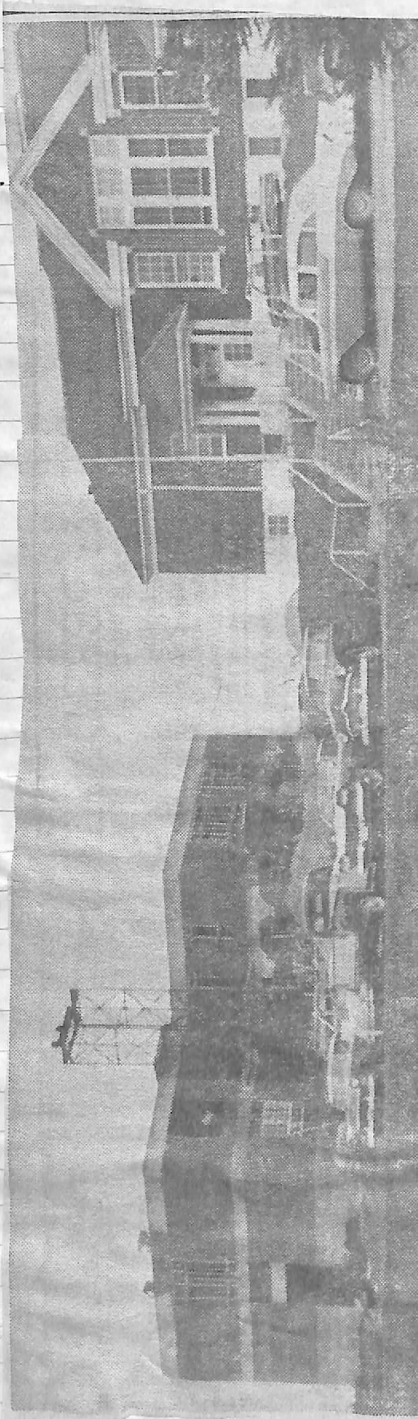
CONSTRUCTION progresses on the second wing at the Monteith Industrial Farm at Monteith. The addition which will hold 120 inmates in four dormitories, with a kitchen and dining room in the basement, is expected to be completed by the end of October. There are now 99 prisoners at the farm but when completed the farm will have a capacity of 240 inmates. (Daily Press Photo)
