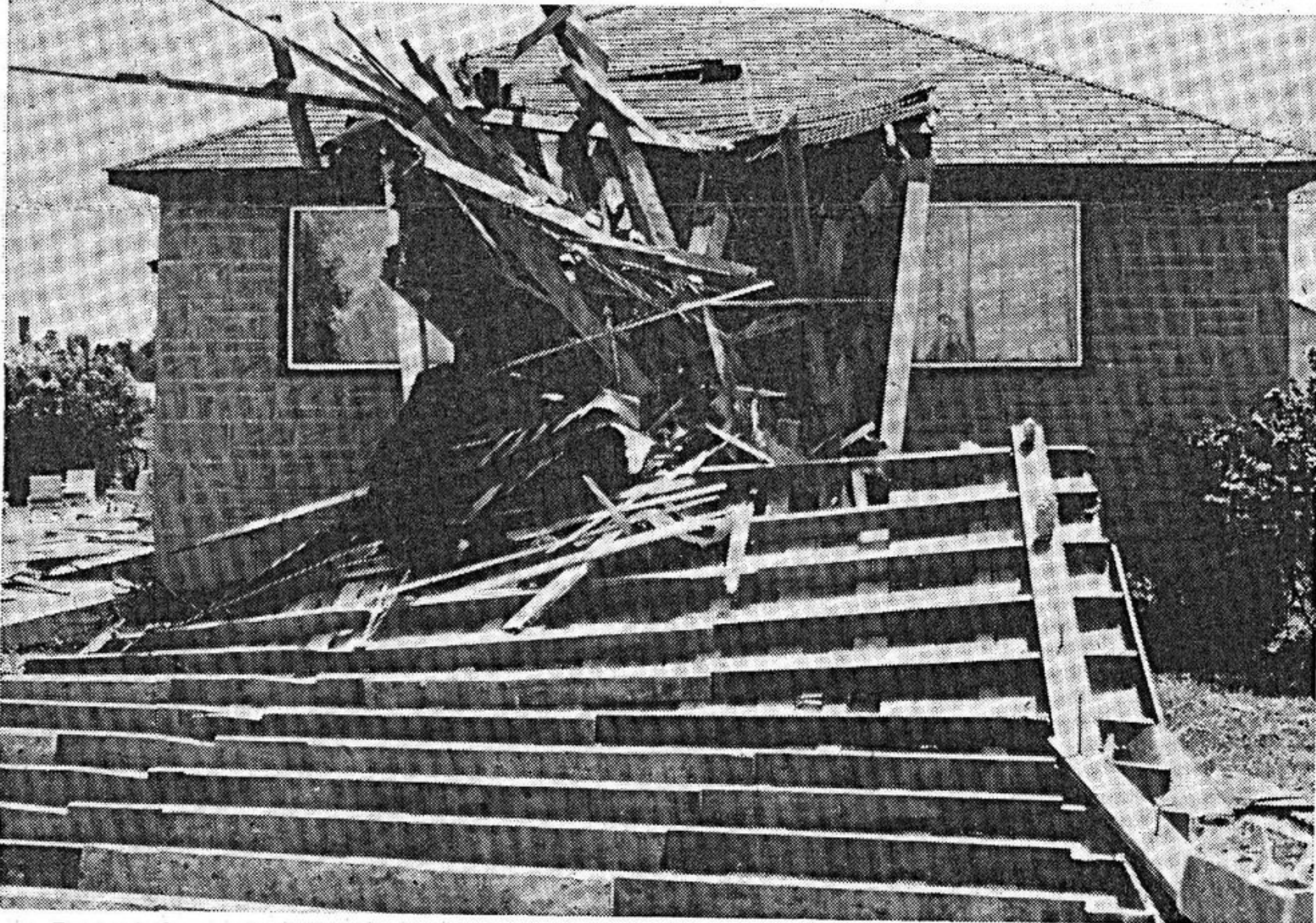
Part of the roof of Renfrew Builders Supplies lies on and in front of the shattered porch at the home of Leslie White on Lisgar street. Total damage from Saturday's storm was estimated at about $15,000.
