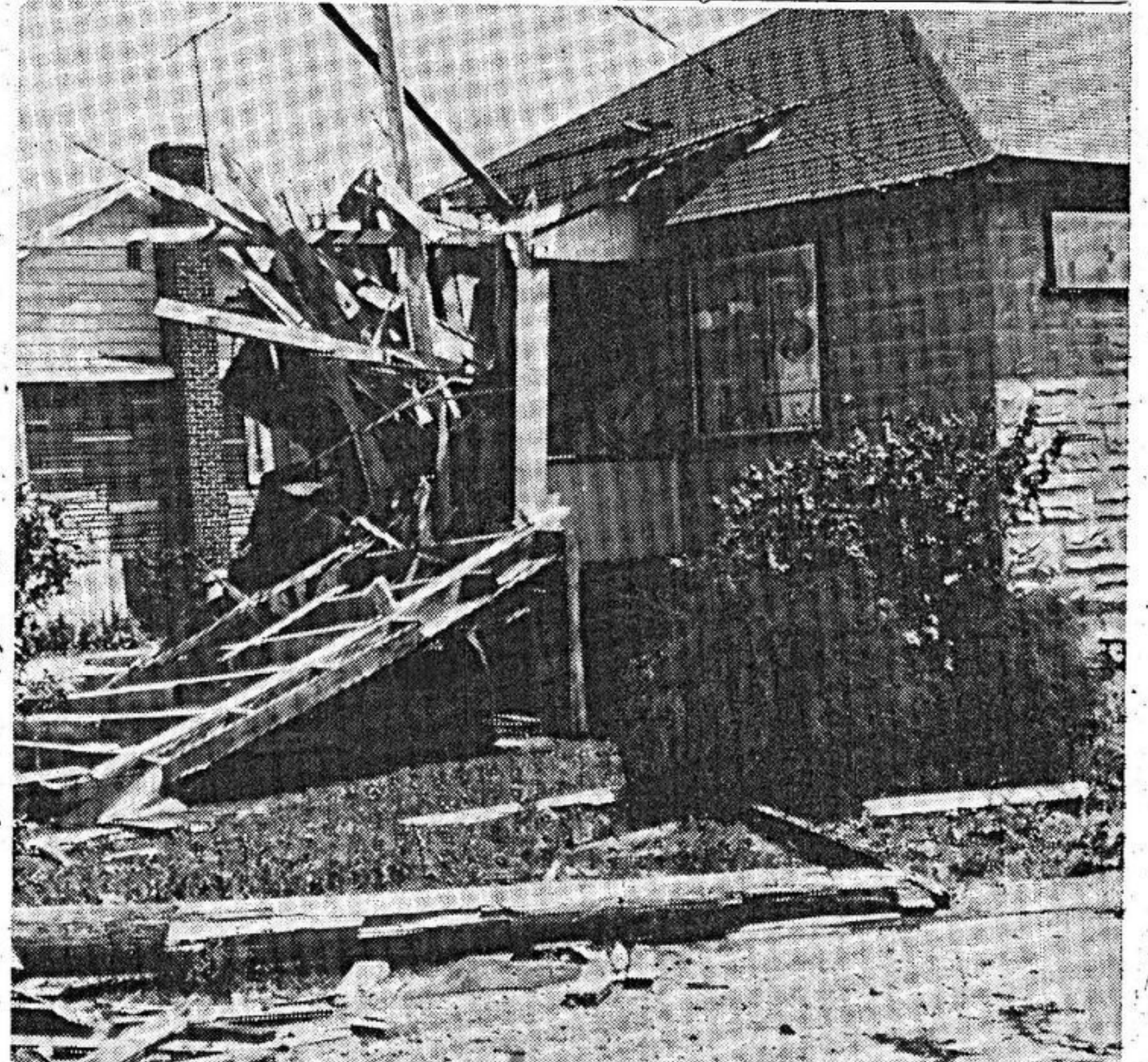
Debris lies scattered before the home of Leslie White on Lisgar street. The porch was smashed by the impact of part of the roof from Renfrew Builders Supplies.
