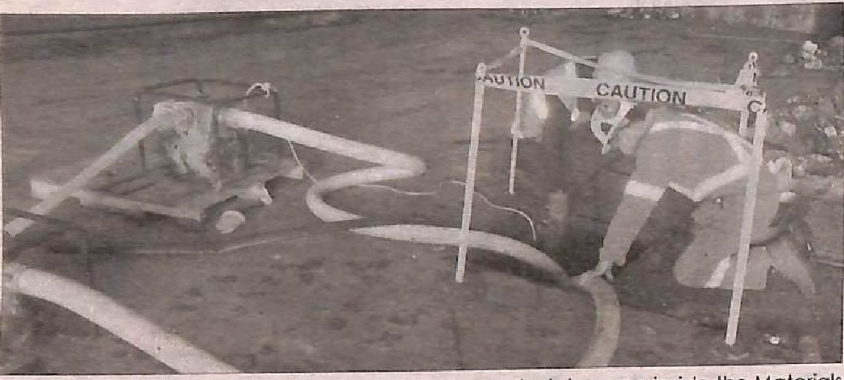
GRAFTON -- Northumberland County officials inspected damage inside the Materials Recovery Facility in Grafton on April 14, after a smoldering fire broke out inside the facility the day before. Staff members are now conducting a review to identify potential causes with foul play not being suspected. --Submitted Photo
