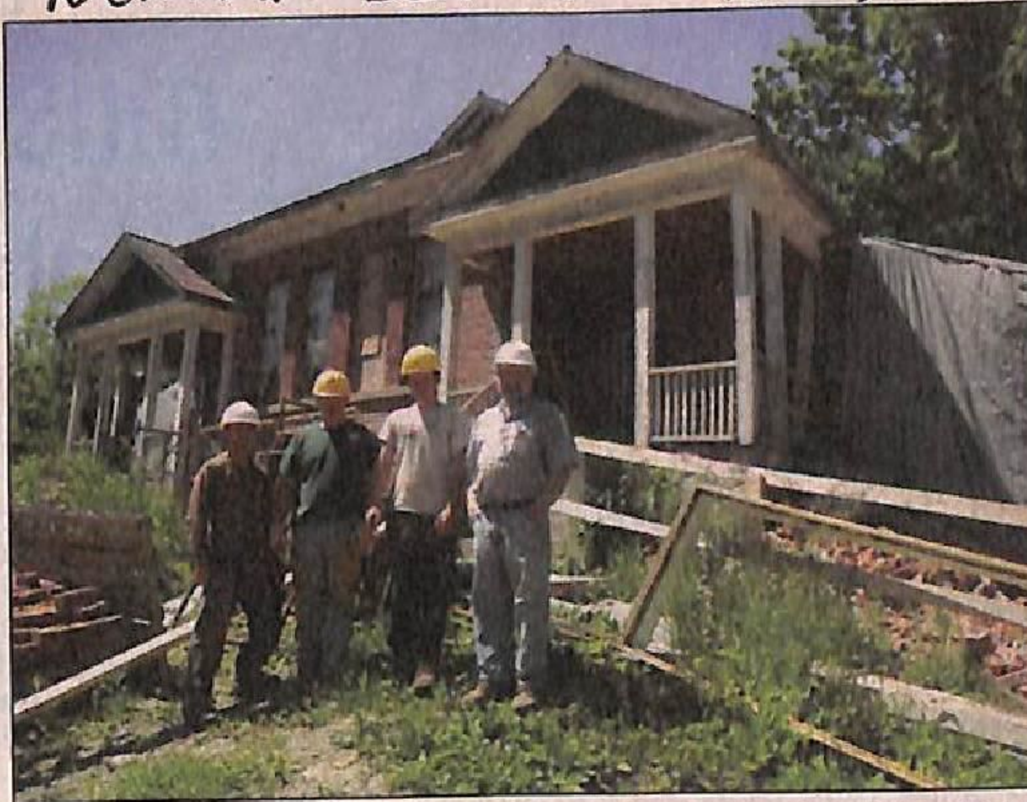
CECILIA NASMITH Northumberland Today (From left) Pat Basinger, Russell Wright, Chris Boot and Rob Green of Green Brothers Construction (seen on June 20) are enjoying the many challenges of restoring this old Centreton schoolhouse.
