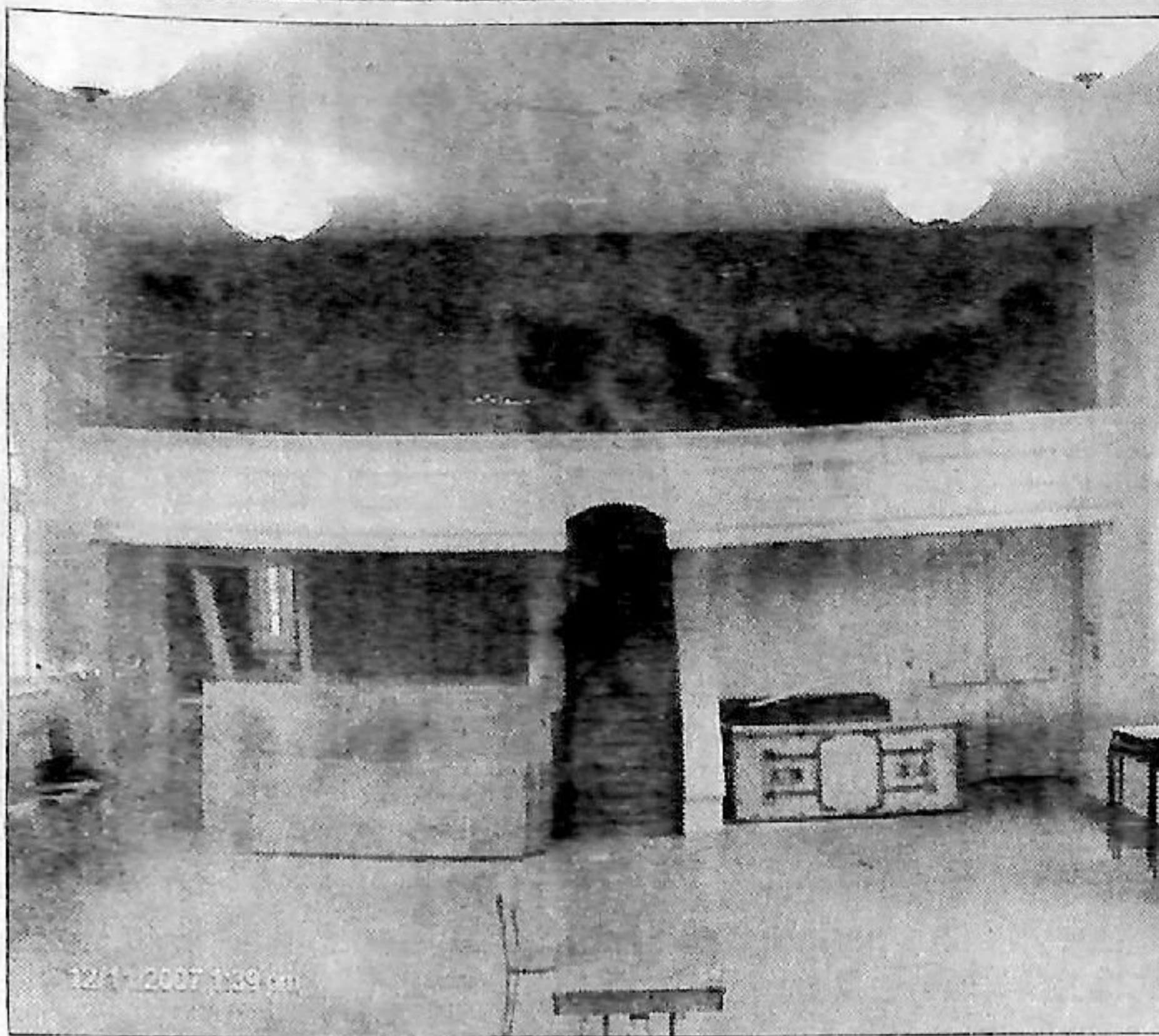
November 2007: The sagging balcony in Castleton
