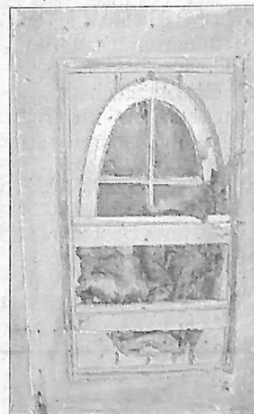
One of several sealed windows in the balcony of Castleton Town Hall has been opened up.
