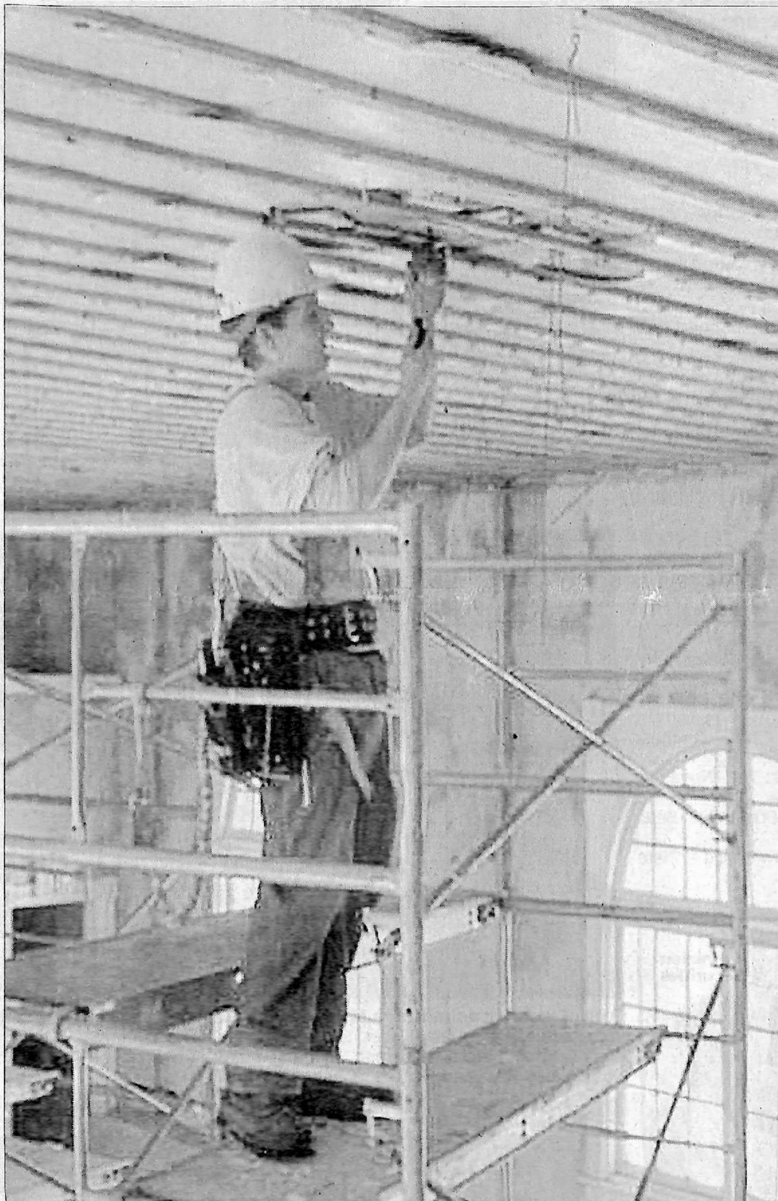
High up under the ceiling electrician apprentice Derrick Vandervelde attends to the preliminary work of phase one of the restoration project.
