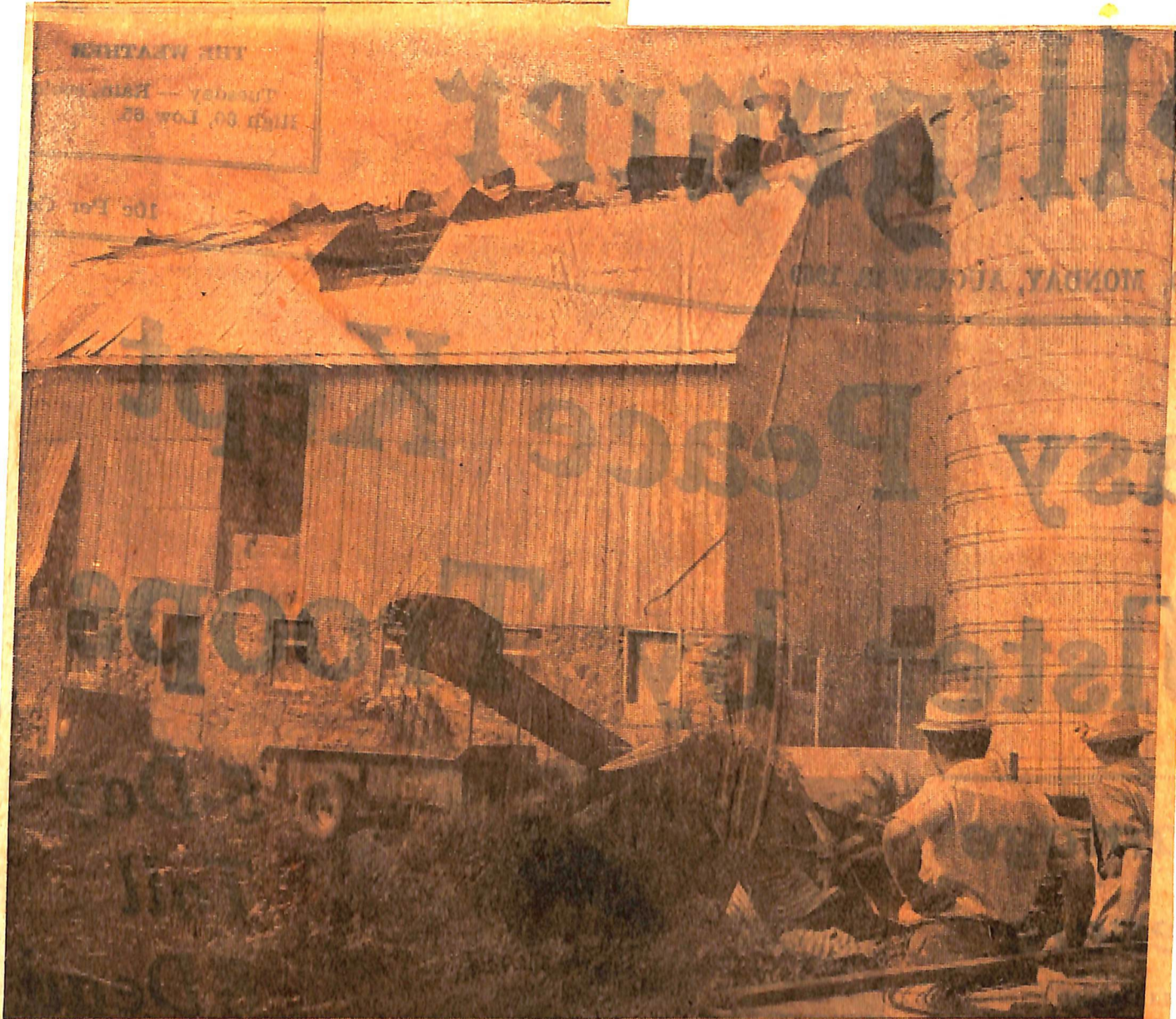
NEIGHBORS OF DOUGLAS SILLS, 9th concession of Thurlow township, view damage wreaked by sudden twister which struck the Sills farm
