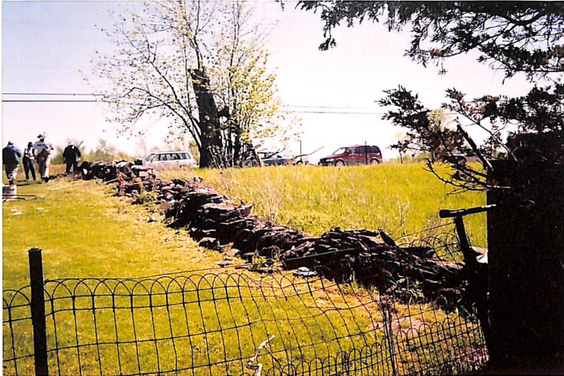
West fence at Pentland in rubble condition
