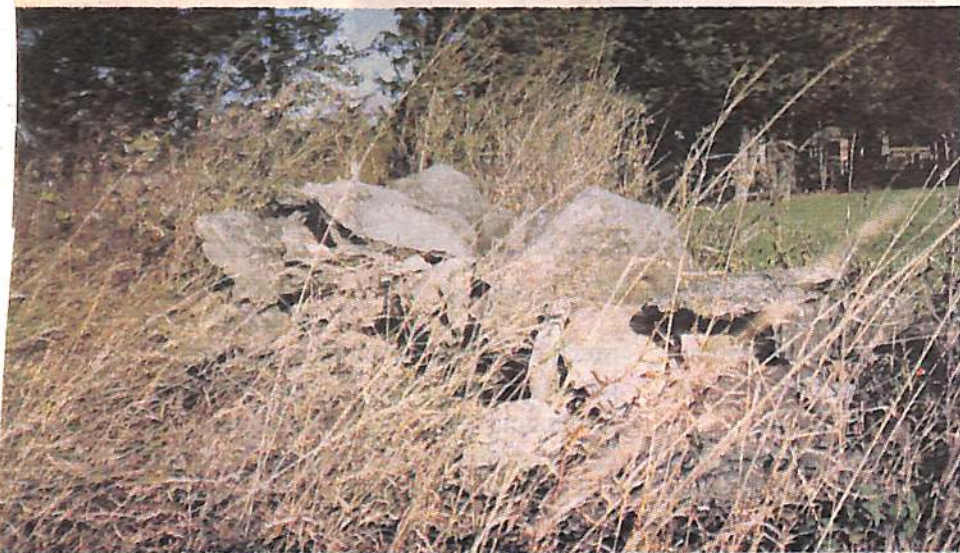
Pentland Fence in need of restoration
