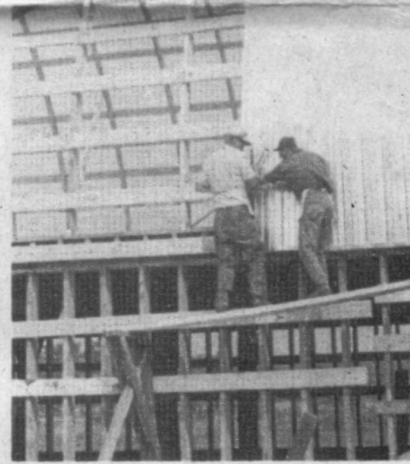
LAYING THE METAL ROOFING ARE, FROM BO top, Percy Runtz, right, Gerald Neill, left, Wilb Billy Laventure, Brian Box, and Blyth Russett.
