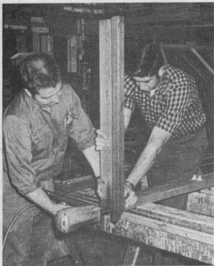
ARTHUR CAMPBELL AND FRANCIS HERBERT assemble a window frame using modern power tools.
