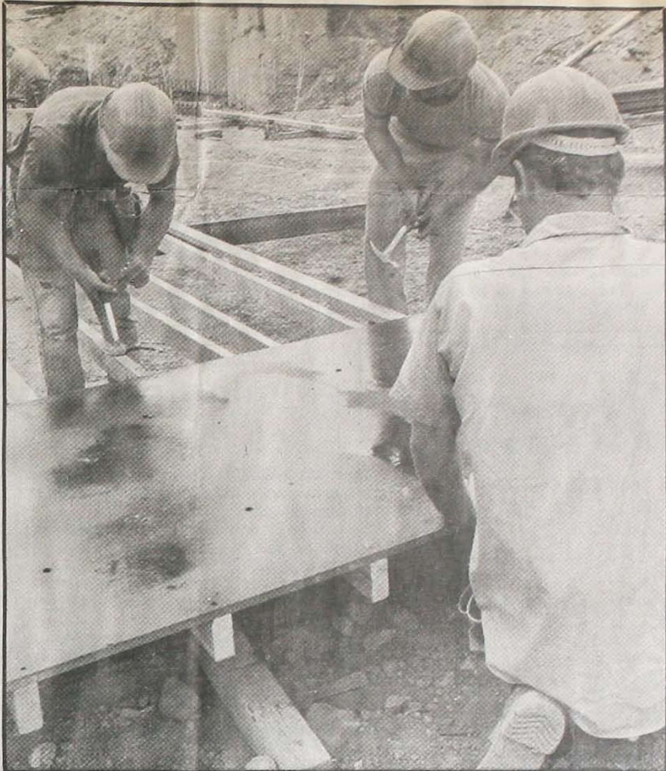
NAILING THE FORM FOR THE SLUICE wall at the Maple Hill Power Station is Murray Grubb (back to camera), Andrew Meyer, left, and Herb Thynne.
