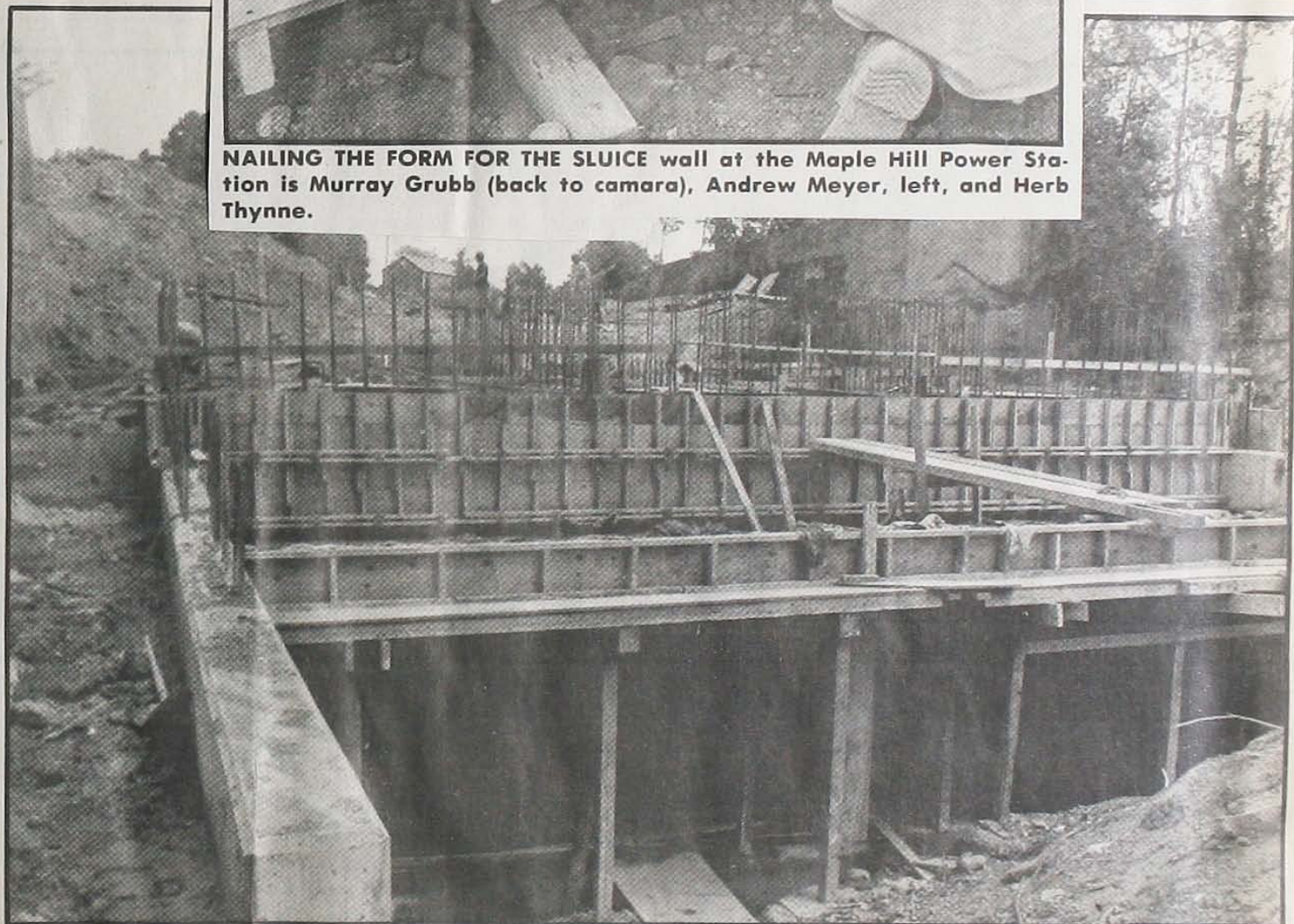
A NEW POWER STATION is being built on an old site of a hydro plant at Maple Hill Dam, east of
