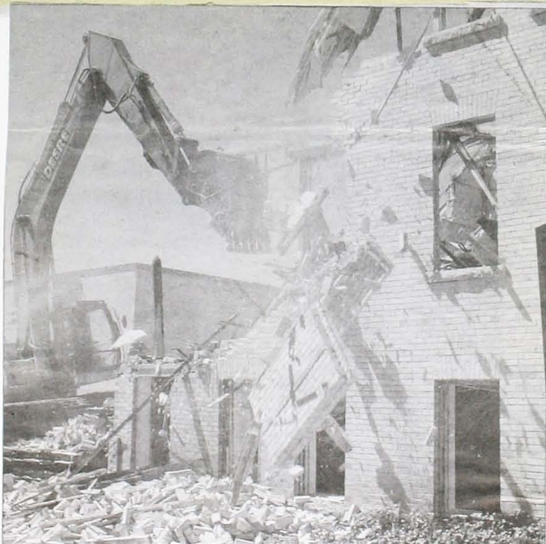
Work crews at the former nurses' residence at the Walkerton hospital began taking the walls down in August. The windows were removed first and all infrastructure disconnected. The demolition was completed around the end of the month, making way for the new Brockton and Area Medical Clinic, which is to be started in 2009.
