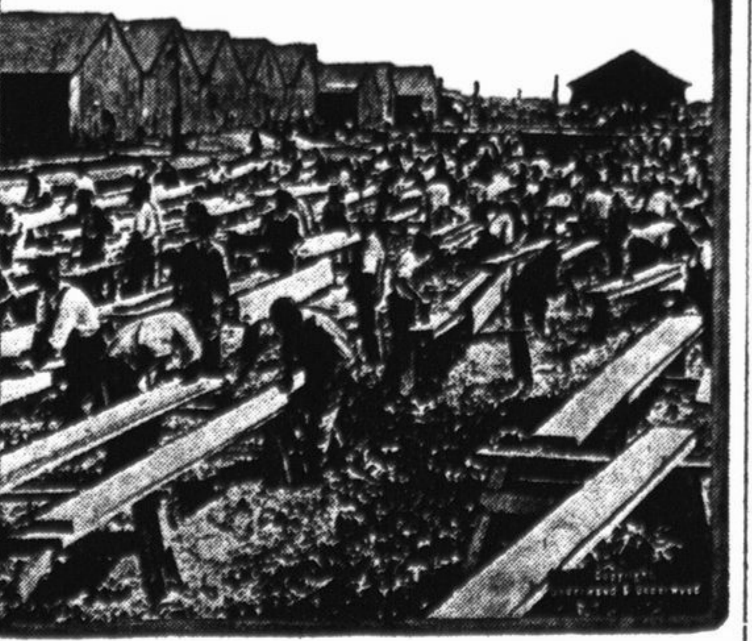
Carpenters working on new hangars at one of the aviation training schools "somewhere in the United States." Each day as more men join the air service the need for greater training camps becomes pressing. Every camp is being enlarged for the great corps of flyers Uncle Sam is training.
