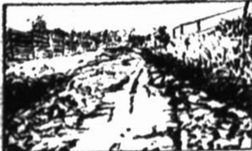
Poorly Located and Badly Drained.
