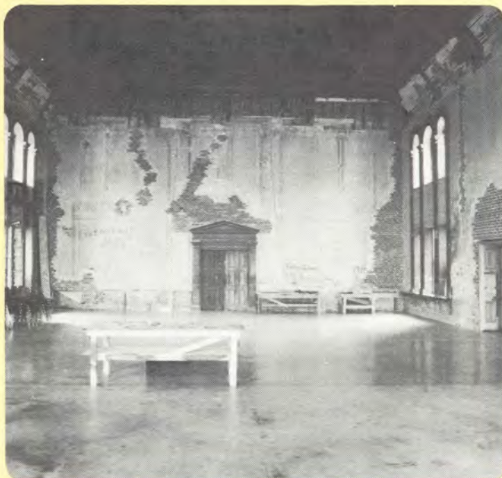
Partial view of Grand Concert Hall to be restored in Phase III.*
