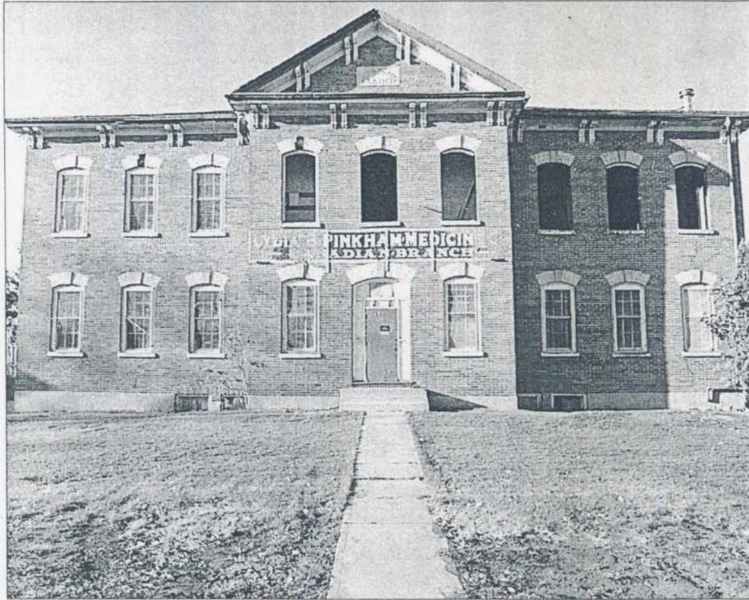
THINGS OF THE PAST: Workers have begun the task of dismantling the Lydia Pinkham building for Whitehall, right, continues.
