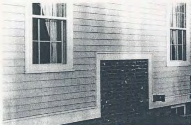
Another device borrowed from the past is the exposed brick wall of the fireplace, a feature which generally disappeared from frame construction by the 1850s. Its inclusion here helps lend the Smith house a pre-Victorian character.
