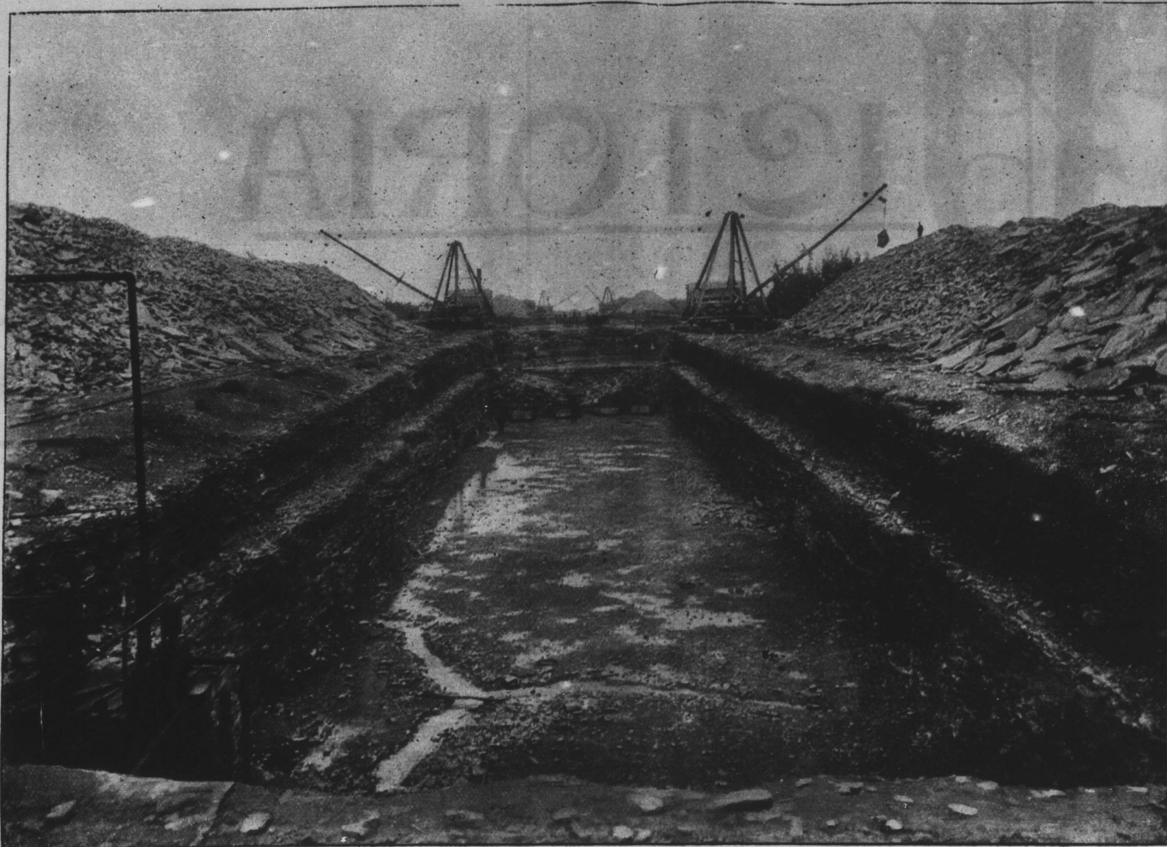
ROCK CUTTING, TRENT CANAL, BETWEEN KIRKFIELD AND VICTORIA ROAD, IN NORTH VICTORIA Station No. 1, showing Station No. 2 in the distance.
