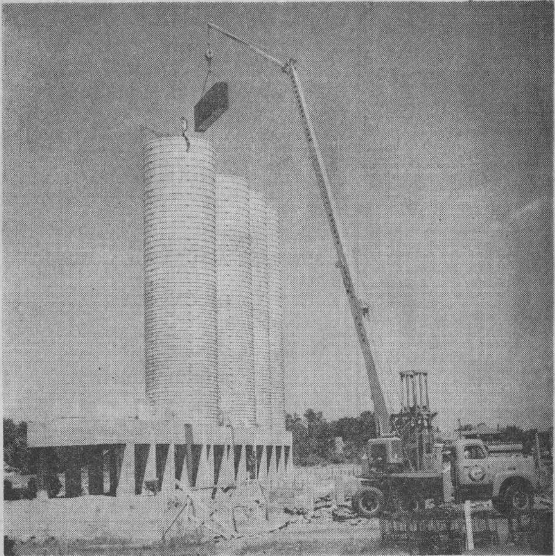
Eight sixty-foot storage silos, four of which are shown above are one of the construction features of the new plant now being built by the Wilson Concrete Products Ltd. on its Sidney Street site. In the foreground is the new mobile hydraulic crane which has a boom extension of 75 feet. The company expects to be in production in early October.
