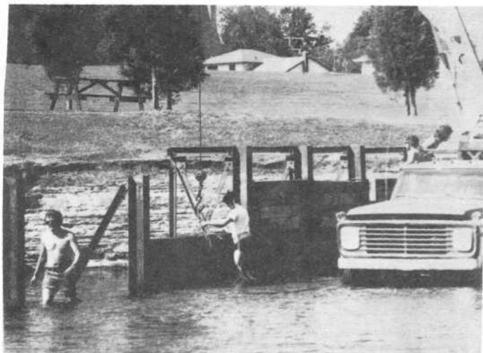
Crew from United Rigging installing seasonal dam at Riverside Park 'Wader' at left is Ray Finkle.
