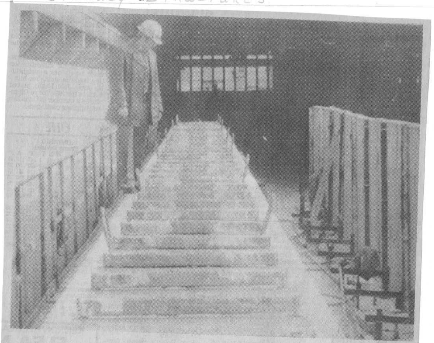
Bill Letman, technical sales representative for Stanley Structures, checks out a fresh pouring of concrete in the form for a 129-foot beam.
