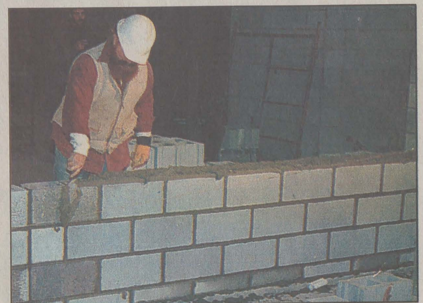
Construction of the new Student/Community/Business Learning Center is moving indoors for the winter.
