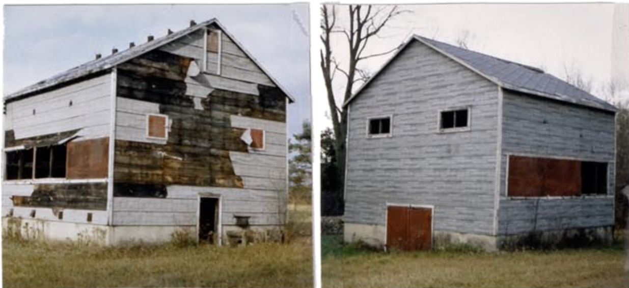
Abandoned kilns at the Yarek place, on the north hill overlooking the millpond at Oakland. This land was the original Malcolm homestead.
