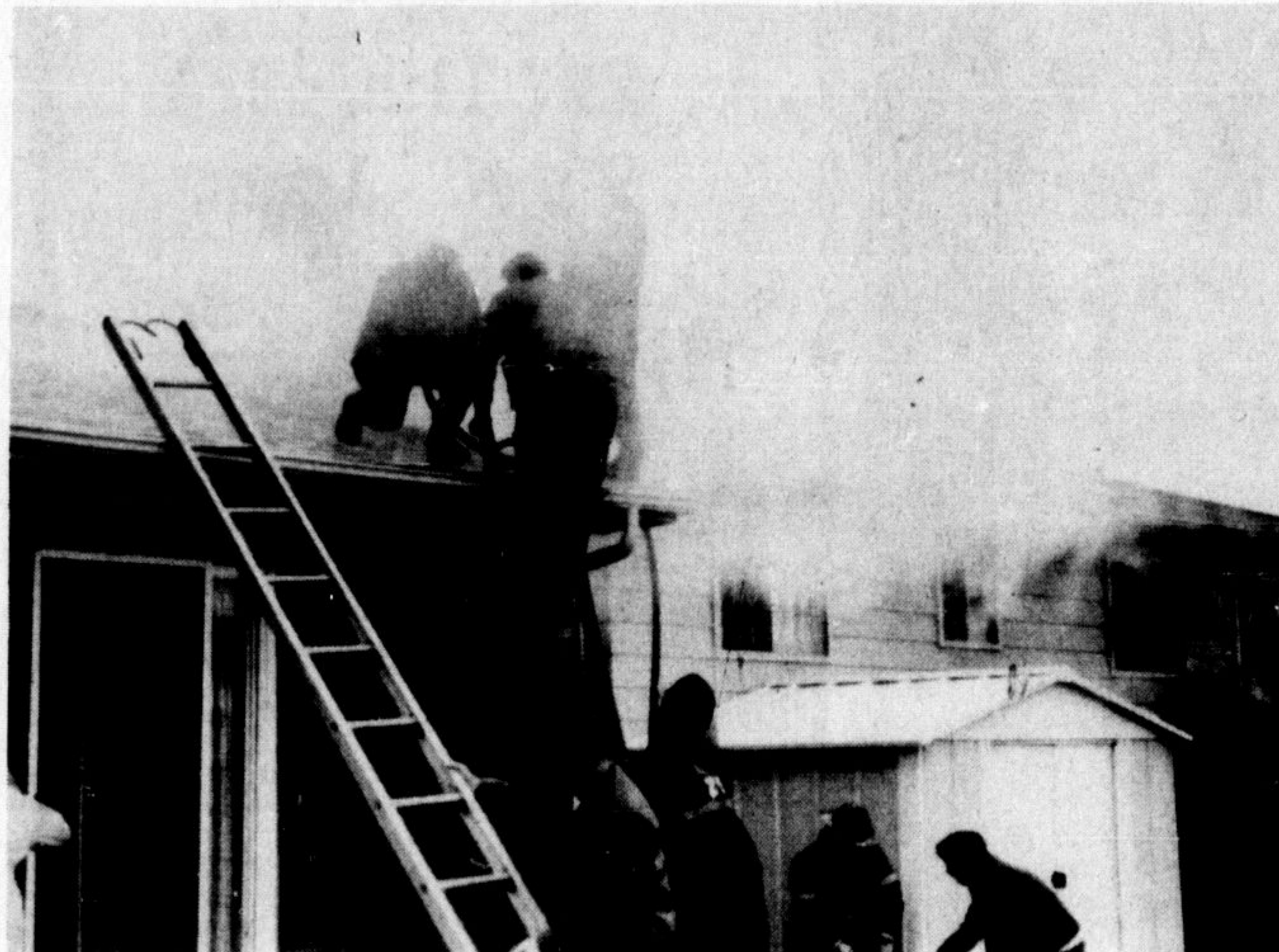
CLIMBING ONTO THE ROOF at the McDonald home on Churchill Ave., early Monday morning, Milton Firefighters received assistance from Dorset Park neighbors. Fire broke out in the area of the home's fireplace, destroying a wall and part of the living room ceiling. Neighbors rushed to the home with hoses before the brigade arrived. Lt. Jim Coulson credits the neighbors with preventing a lot more damage. Cost of damage and the cause are not yet known.
